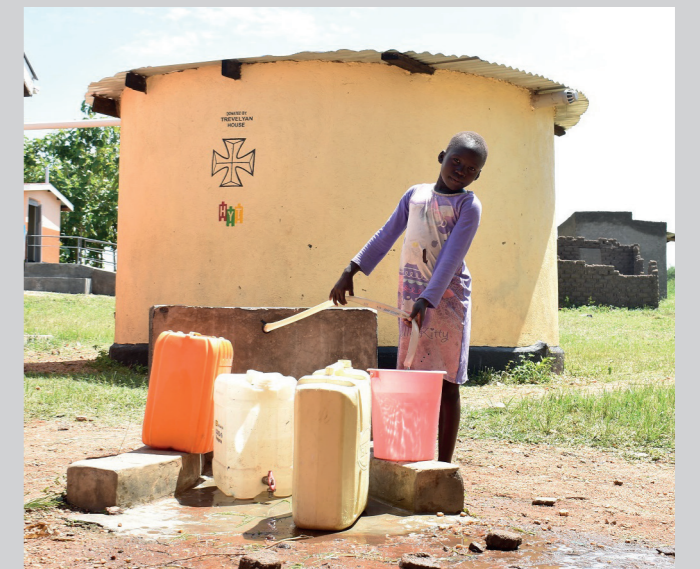
20,000 litre rainwater harvesting tank in Bidi Bidi refugee settlement that was donated by Trevelyan House
